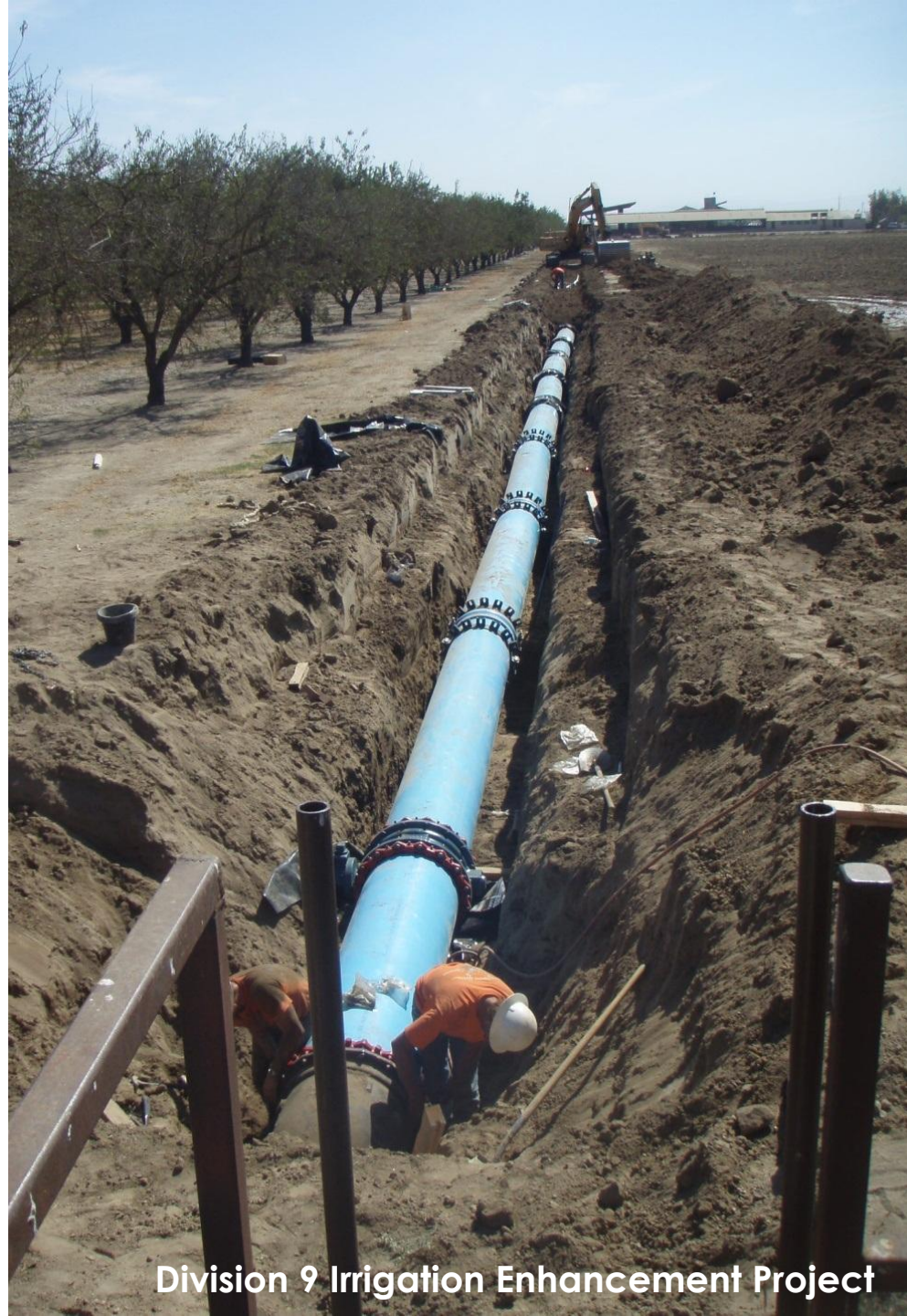
AWWA Class Pipeline Components
