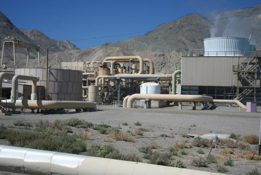
Geothermal power plant
