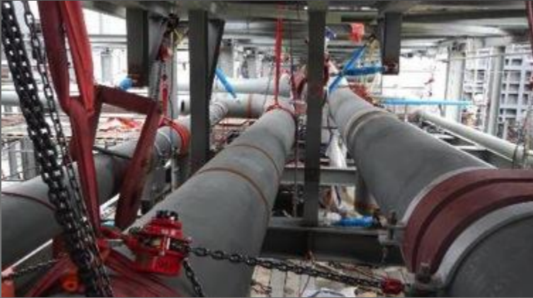
Main rack salt pipe
